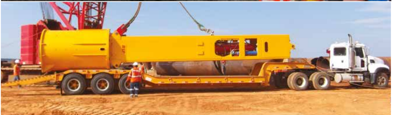
TOP: BSP DX-SP Hammer, excavator mounted, driving sheet piles, Whatlington, East Sussex, UK.
